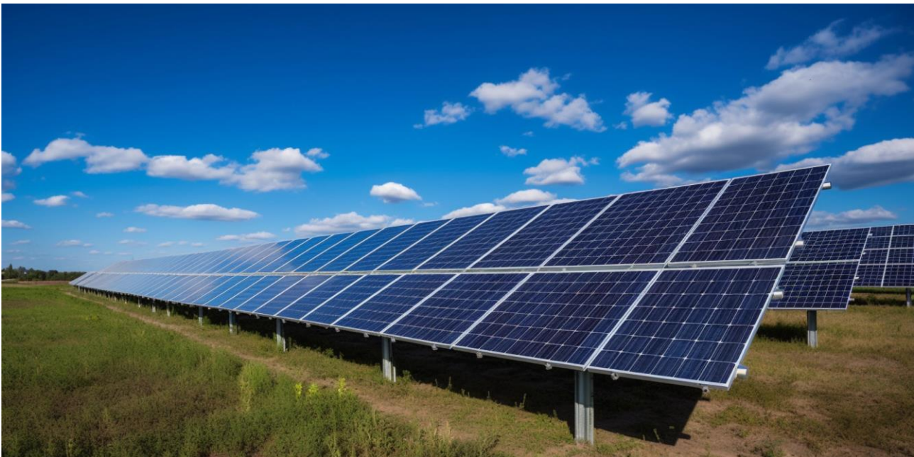
Figure 5.2 Indicative Solar Array and mounting structure
