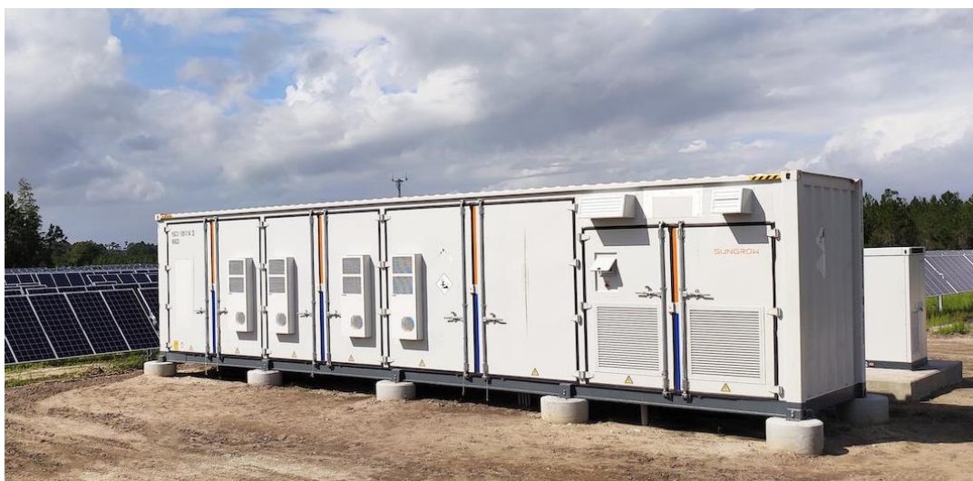
Figure 5.4 Typical BESS Container Example
